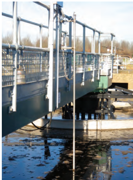
VIPER TRANSDUCER ON CONDUIT WITH ROTATING BRIDGE
